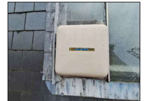
IMAGE 4 THE EXISTING MECHANICAL EXTRACTION FAN UNITS ARE IN POOR CONDITION AND ARE NOISY WHEN IN OPERATION.
