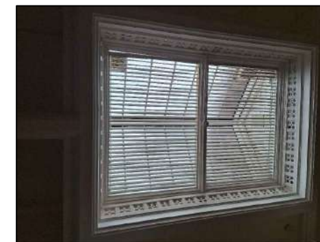
IMAGE 5 VIEW OF THE EXISTING LANTERN FROM WITHIN THE OLD COURTROOM BENEATH AND WITH MODERN SURROUND AND LOUVRE BLINDS AT CEILING LEVEL.
