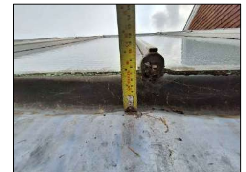
IMAGE 6 THE EXISTING ROOF LANTERN PROJECTS ABOVE THE SLATE COVERING BY 100mm.
