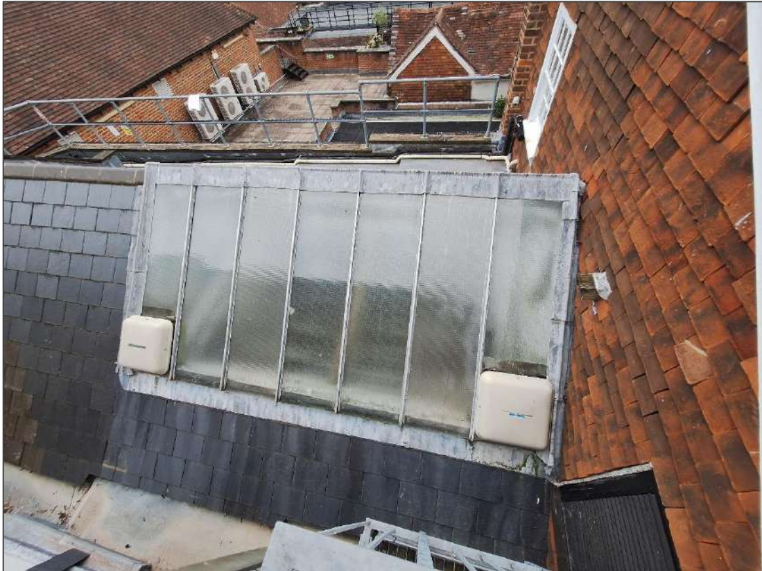
Image 7: The existing roof lantern as viewed from the North side. The wired glass and tired looking mechanical vents detract from the visual appearance of the Listed Building.
