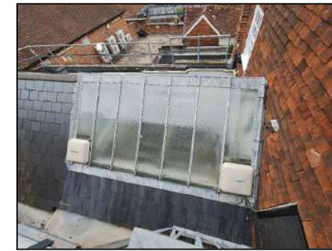
IMAGE 1 VIEW OF THE EXISTING ROOF LANTERN FROM THE NORTH SHOWING EXISTING MECHANICAL VENTS.
