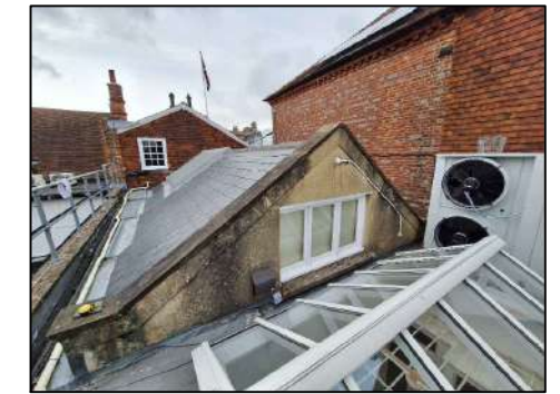
IMAGE 2 VIEW TOWARDS THE EXISTING ROOF LANTERN FROM THE EAST WITH THE RECENTLY REPLACED LANTERN IN FOREGROUND AS APPROVED UNDER APPLICATION 19/00144/LBC.
