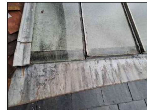
IMAGE 3 THE EXISTING WIRED GLASS IS BEGINNING TO FAIL AND SLIP FROM THE HOUSINGS. THE GLASS IS IN A WORN CONDITION AND BEYOND ITS USEFUL LIFE EXPECTANCY.
